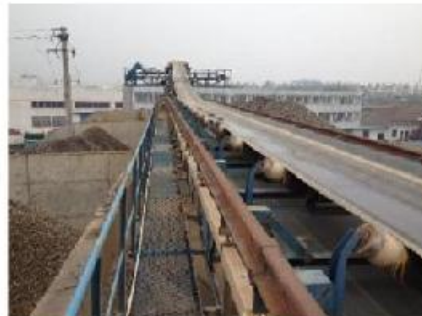
Gambar 35. Coal Handling Unit (Sumber: Ducon)
