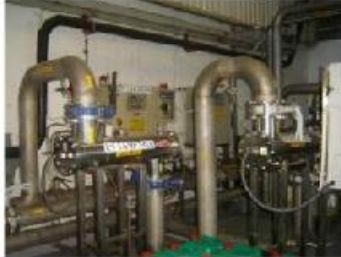
Gambar 34. Chlorination Plant (Sumber: Halmar)
