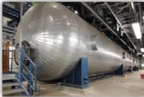
Gambar 25. Boiler (Sumber: General Electric)
