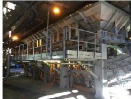
Gambar 36. Ash Handling Unit (Sumber: LGM Industries)
